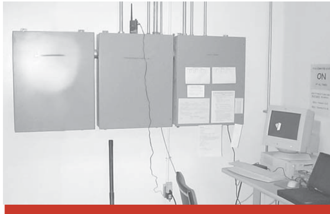
Operational SURE CURE Computer System
