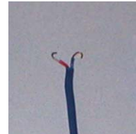
Unshielded wire, stripped and bent.
